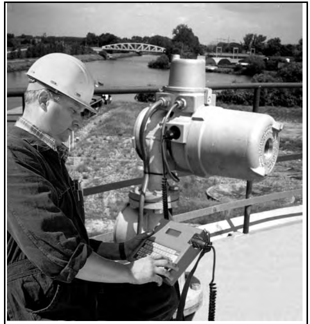
Figure 3.5 Programming the 854 ATG by using The 847 Portable Enraf Terminal
