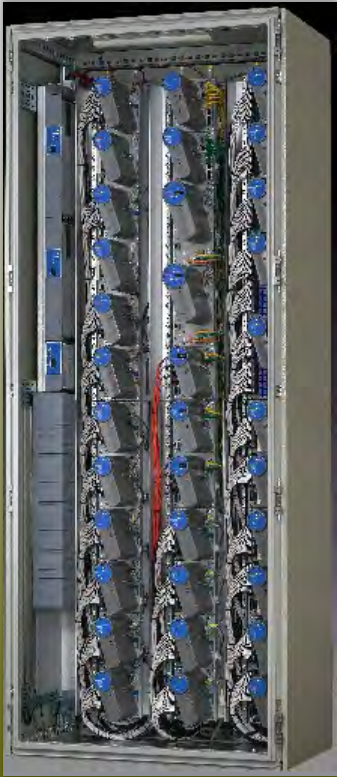
Series C HPS factory built
