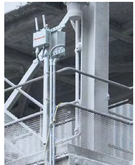
Wiring is a chronic weak point close to a harsh steel furnace.
